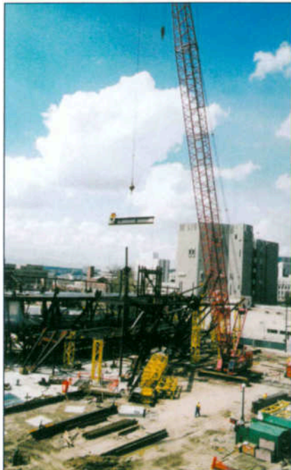
Left and below: By early spring 2004, the complex process of steel erection was well under way. LPR Construction employed a big Manitowoc 888 for the primary erection and a host of extendable boom lift trucks for secondary work. Yellow towers are temporary supports for structural components. Across the street is the main Denver Art Museum, housed in a once-controversial tower designed by architect Gio Ponti. Hol Wagner photos
