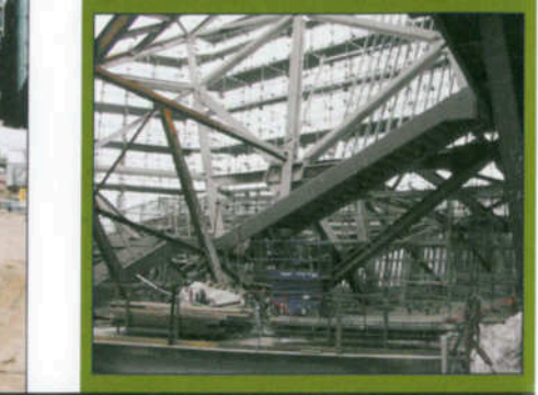
Below: With steel erection completed and skin placement under way, the addition's atrium is a complex mass of girders and beams. M.A. Mortenson photo
