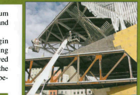
Above: Metal studs for the exterior skin are applied to the prow jutting out over 13th Avenue in this Dec. 15 view. Overhead walkway crossing the street will link the original building to the new addition. M.A. Mortenson photo
